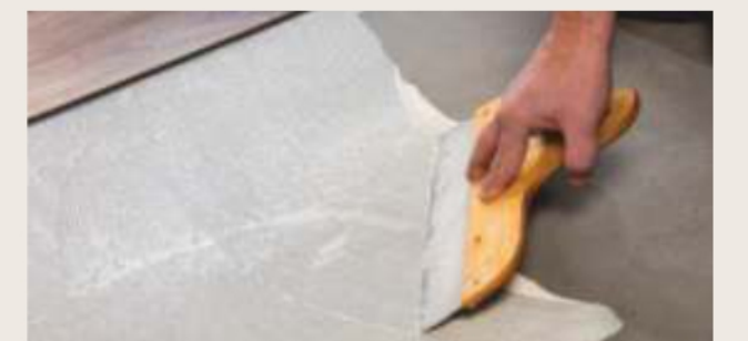
Cracking at corner & around cuts may be caused by improper conditioning, improper bonding, poor planning, avoid all these to prevent cracking at corners.
